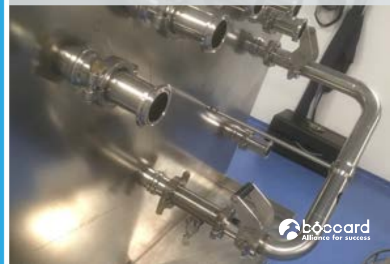
Transfer panel converted to BocLock version (use of clamp / BocLock adapters) to keep the original TP
